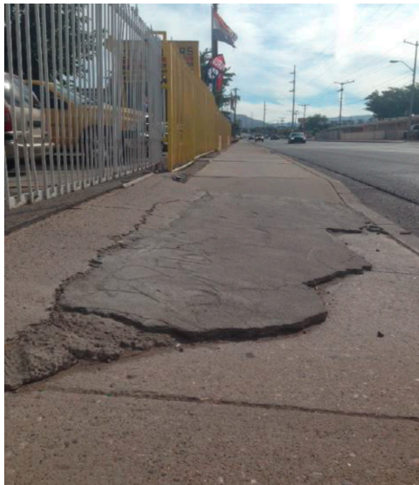
Figure 8. Poorly maintained sidewalk in Z 8.
