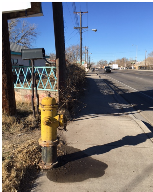
Figure 13. Bridge Boulevard's unused curb cuts and deteriorating infrastructure lowered its scores (B 8).
